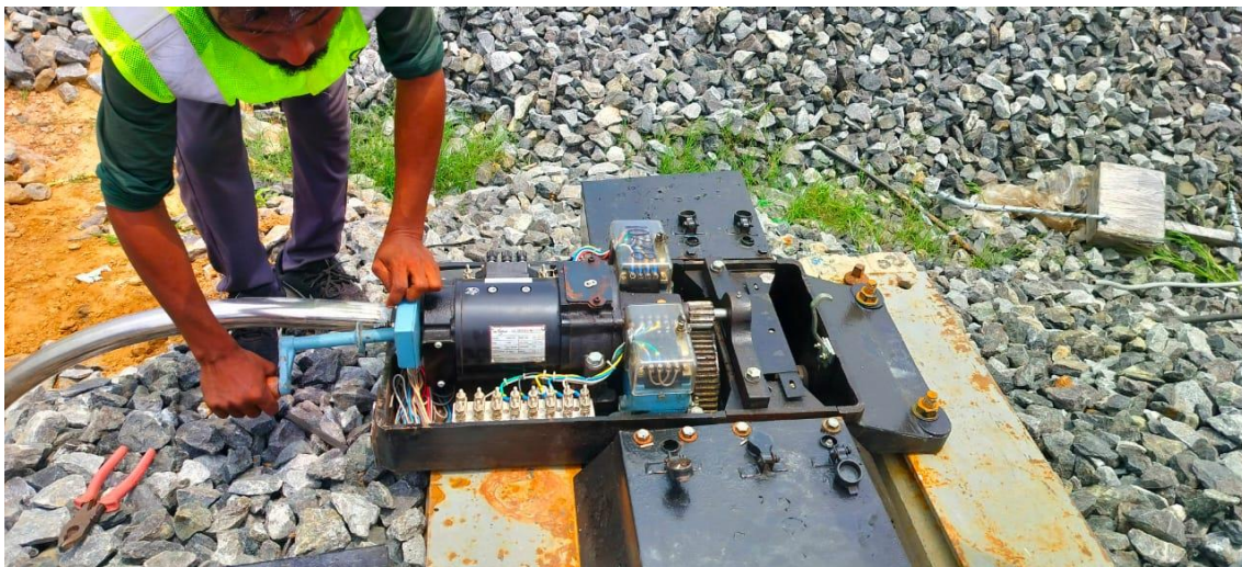
Figure 6. Point Motor is used to change the direction of Train Movement.
