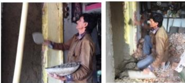
(i) (ii) (c) Applying mortar on the wall (for inside plastering) (PL-3)
