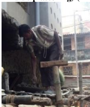
(e) Picking mortar for Plastering (to apply on the wall) (for outside Plastering) (PL-5)
